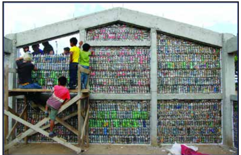
Kids in San Martín Jilotepeque Guatemala, help collect and stuff plastic bottles to make ecobricks, which are used to build the walls of these schools. Photo credit: Hug It Forward
