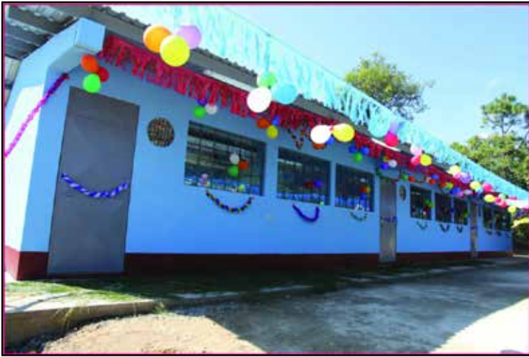
Once in place, bottles are covered with a layer of cement and the new walls are painted to create colorful classrooms. Photo credit: Hug It Forward
